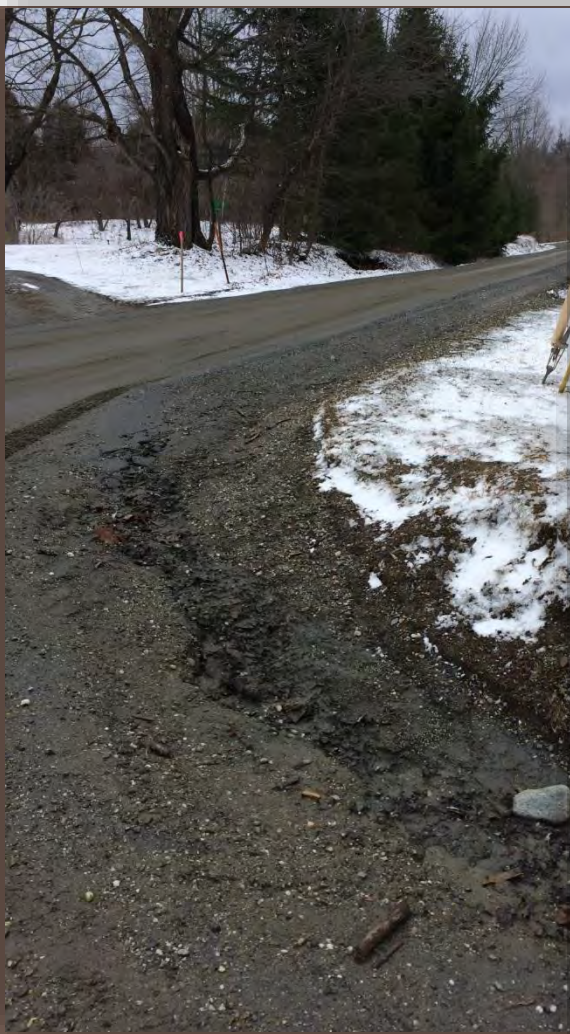
Road Runoff Causes Maintenance Issues
