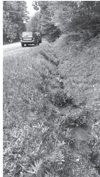
Kew Vasseur Road: Note over-widened road and steep, eroding ditch full of sediment.
